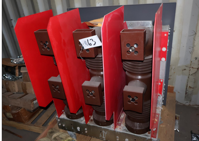
EATON 380VPCW-HDR25 38KVS MEDIUM VOLTAGE VACUUM CIRCUIT BRAKER
