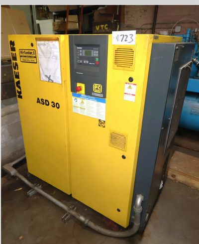
KAESER ASD-30 30HP SCREW TYPE AIR COMPRESSOR
