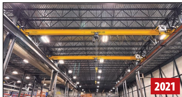
2021 FRONTENAC 40' X 200' FREE-STANDING CRANE SYSTEM
