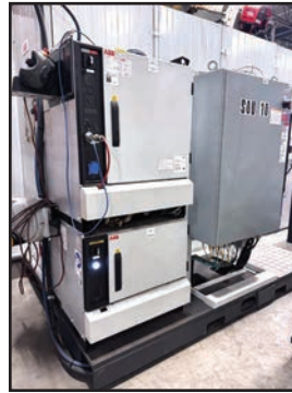
VIEW OF ABB IRC5 ROBOT CONTROLS
