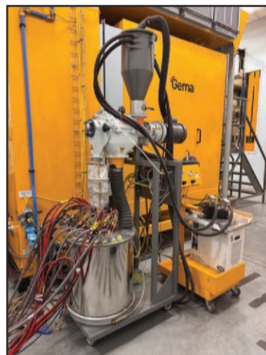
GEMA RECLAIM SYSTEM
