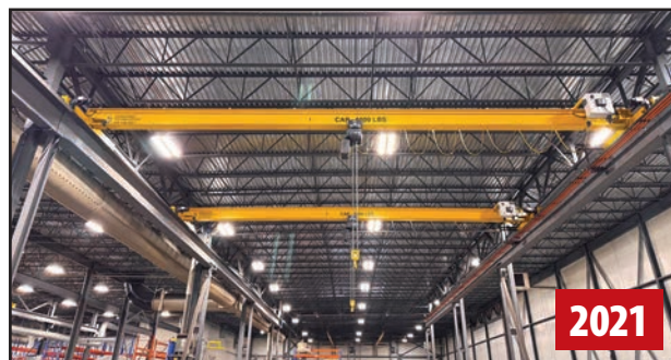
FRONTENAC 40' X 200' FREE-STANDING CRANE SYSTEM
