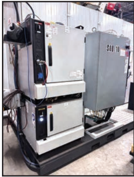
VIEW OF ABB IRC5 ROBOT CONTROLS
