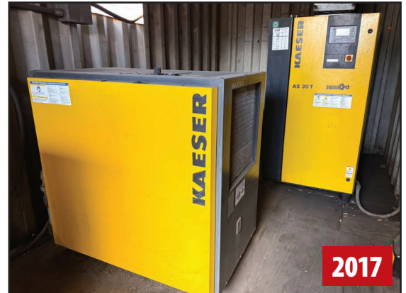
KAESER 30 HP ROTARY SCREW COMPRESSOR & DRYER
