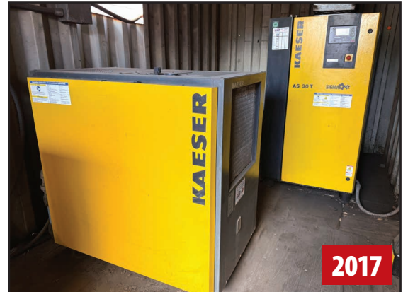
KAESER 30 HP ROTARY SCREW COMPRESSOR & DRYER
