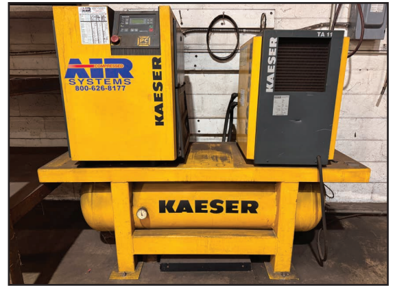
KAESER SM11 10 HP ROTARY SCREW COMPRESSOR/DRYER
