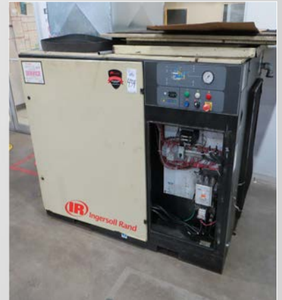
INGERSOLL RAND UP6- 50PE-125 ROTARY SCREW AIR COMPRESSOR
