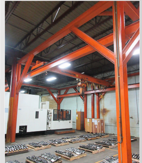
HARRINGTON 3-TON FREE STANDING OVERHEAD BRIDGE CRANE
