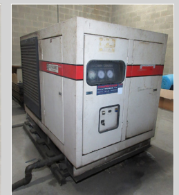
GARDNER DENVER ELECTRA-SAVER II ECMQLB 75HP ROTARY SCREW AIR COMPRESSOR
