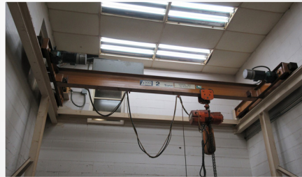
ACCO 2-TON BRIDGE CRANE
