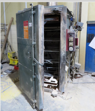
CONTROLLED PYROLYSIS PTR5NT2799 GAS FIRED CLEANING FURNACE
