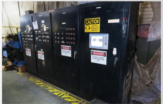
EISENMANN 5-STAGE WASH TREATMENT SYSTEM
