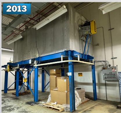
2013 NATURAL GAS-FIRED PAINT CURING OVEN
