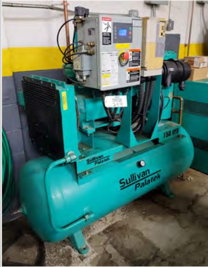
SULLIVAN PALATEK 15DVFD AIR COMPRESSOR
