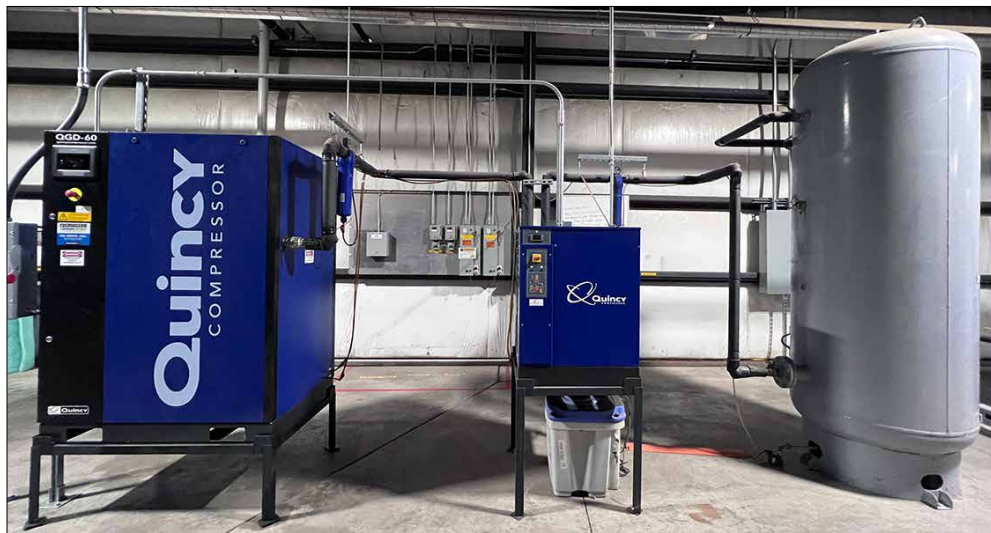
Quincy OGD-60 60-HP Rotary Screw Air Compressor
