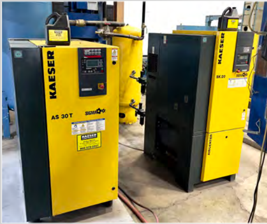
KAESER AS30T AIR COMPRESSORS
