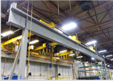
R & M FREE STANDING BRIDGE CRANE
