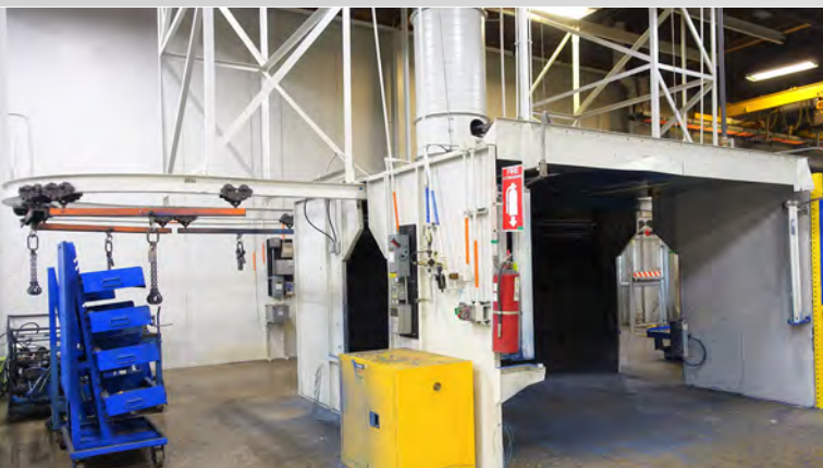
DEVILBISS PAINT ARRESTOR TYPE SPRAY BOOTH
