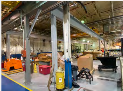
10-TON PIEDMONT HOIST & CRANE
