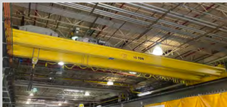
15-TON PIEDMONT HOIST & CRANE
