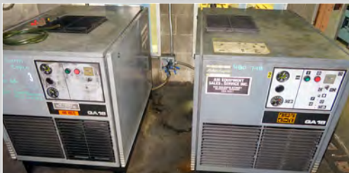
ATLAS COPCO GA-18 AIR COMPRESSORS
