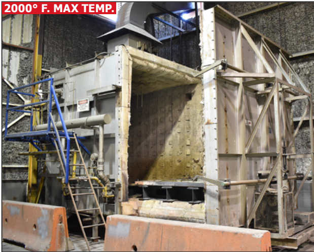
CANFCO car bottom natural gas fired heat treat furnace
