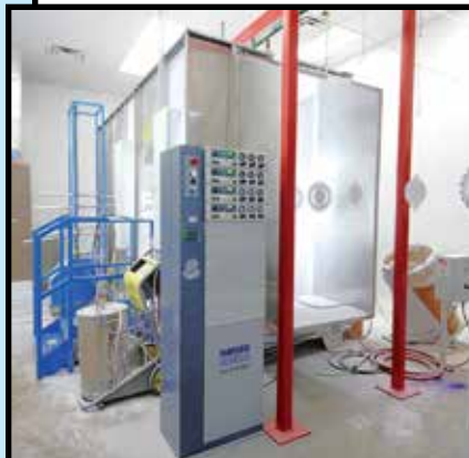
PARKER IONICS RECIRCULATING POWDER COAT BOOTH
