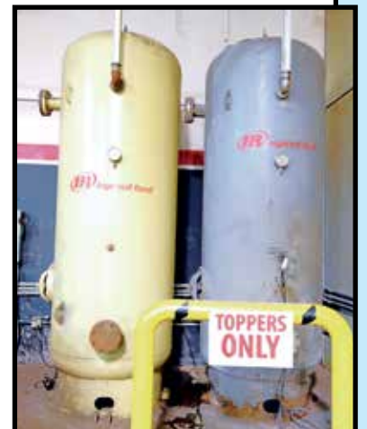
AIR RECEIVER TANKS
