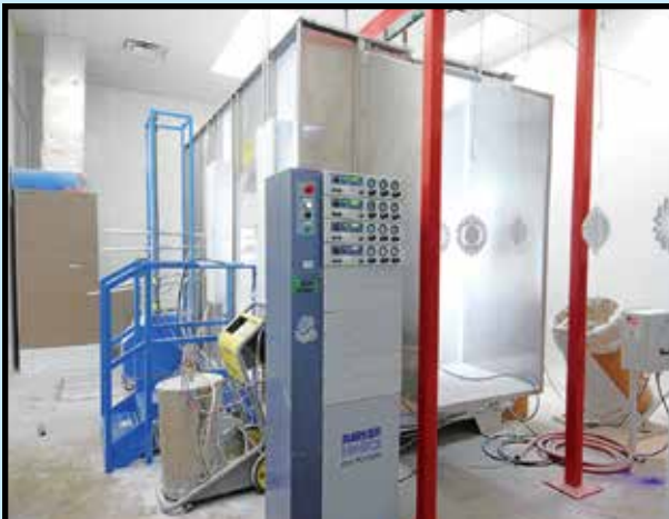
PARKER IONICS RECIRCULATING POWDER COAT BOOTH
