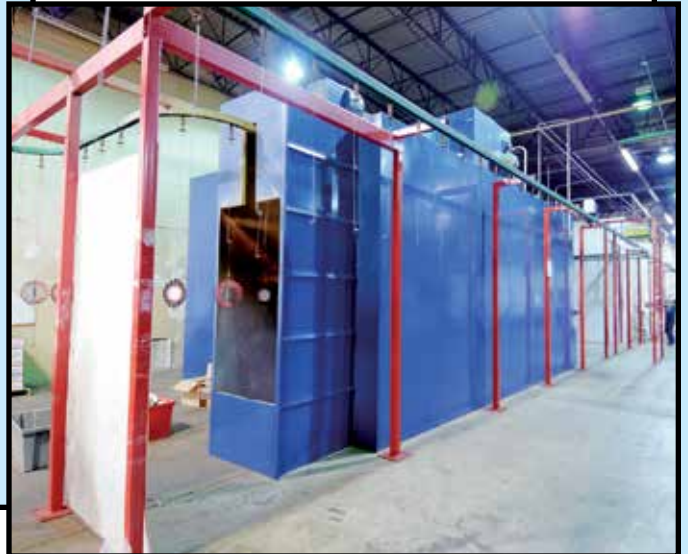
GENERAL AUTO. TRANSFER 2-PASS GAS FIRED OVEN
