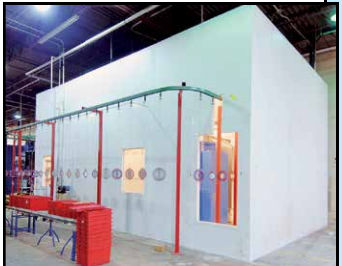
OVERALL VIEW OF POWDER COAT SYSTEMS
