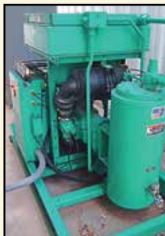
SULLIVAN PALETEK 50 HP AIR COMPRESSOR
